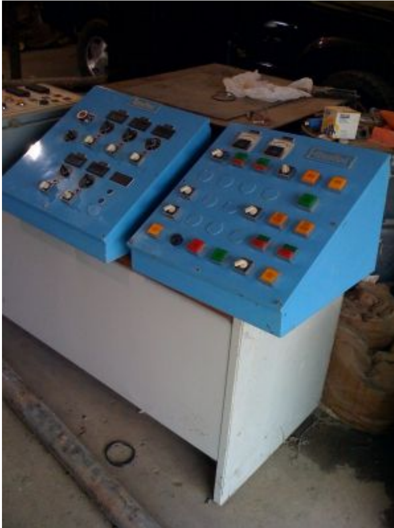
Coastal Control Boxes.jpg
