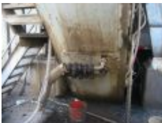
IMG_3511 oil line.jpg
